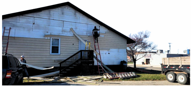
Above: Workers replace the siding on the Vodec duplex in Council Bluffs.
