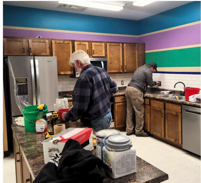
Above left to right: Lindell Construction Owner Dale Lindell and a construction worker remodeling the kitchen in the Cares program in Omaha.
